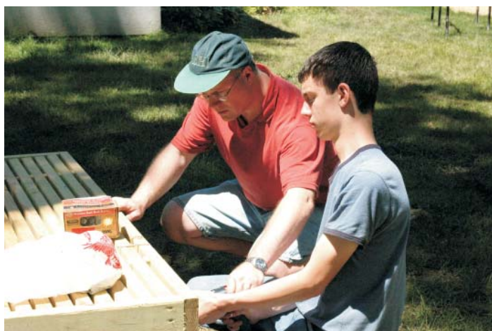
Ryan Stirrup works with his dad in putting the finishing touches on the fire pit project he has developed as part of his Eagle Scout requirements.
